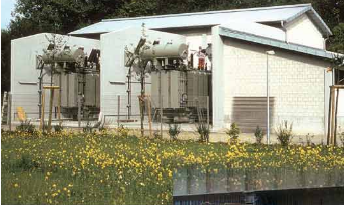
Application Public power supply system
